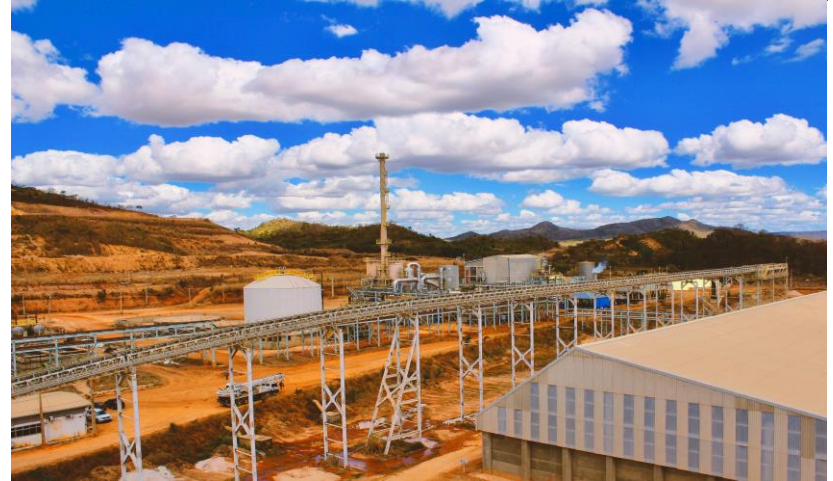
Sulfuric acid plant
