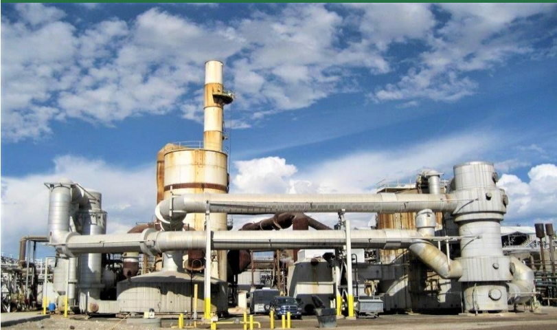
Sulfuric acid plant
